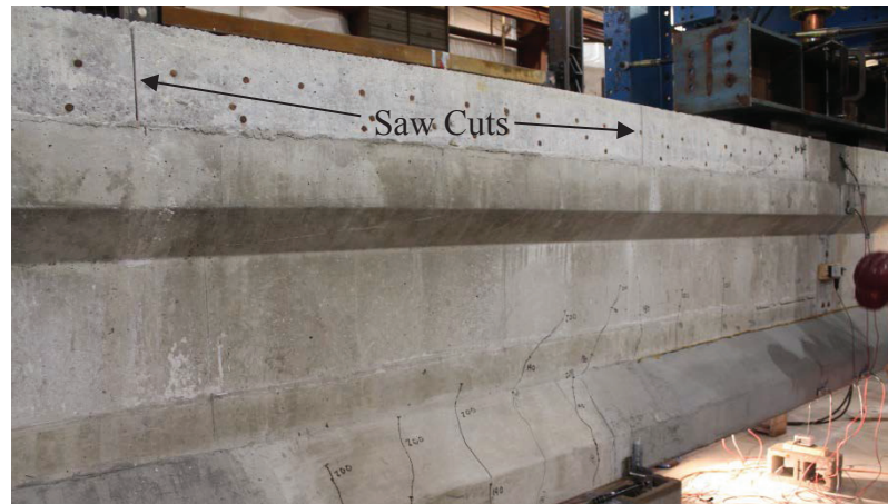
Figure 40 – Saw Cut Gaps in Concrete Deck of Girder D
