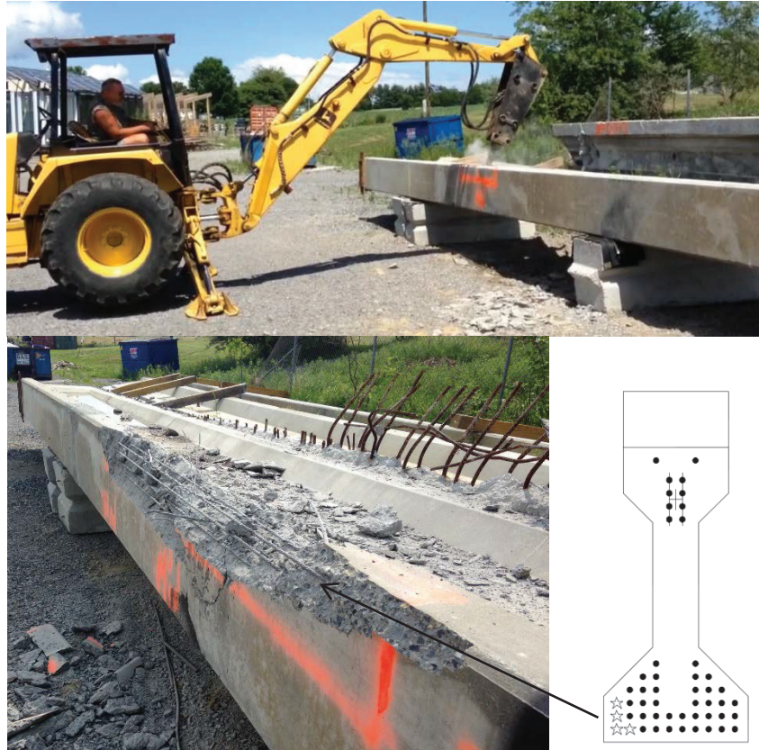
Figure 45 – Prestressing Strand Damage
